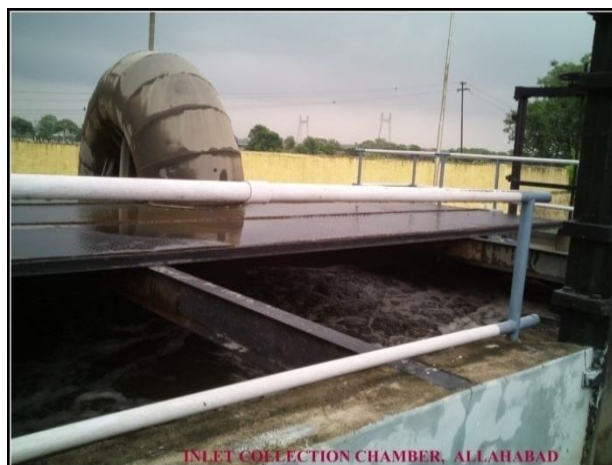
Fig-4: Pictorial represent of inlet (raw sewage) at Naini, Allahabad
