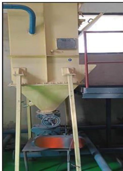
Fig 2: Feed station and Discharge valve
