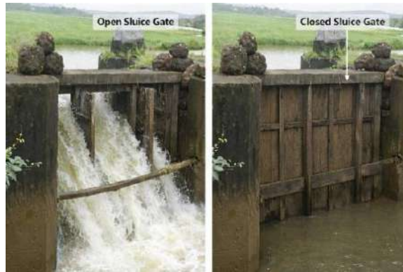
Figure3: Sluice Gate (Manos)
