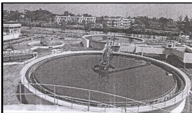
Primary Settling Tanks
